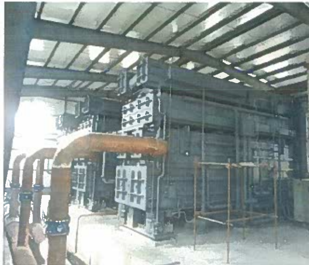
3 x 30 MW Absorption Heat Pumps for District Heating application at Harbin, China
