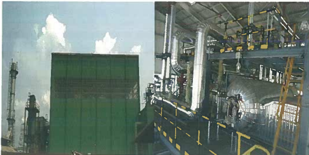
A Cogeneration boiler for our customer in the Democratic Republic of Congo (DRC), Africa
