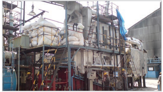
1 X 50 TPD Pilot Plant at Thermax R&D facility
