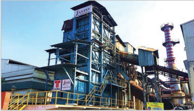
1 X 75 TPD MSW fired hot gas generator
