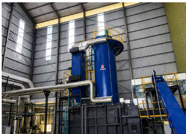
The biomass-fired reciprocating grate thermal oil heater installed at the glove manufacturing site
