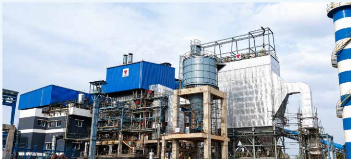
The 1 x 47 TPH AFBC boiler installed at the grain-based ethanol distillery
