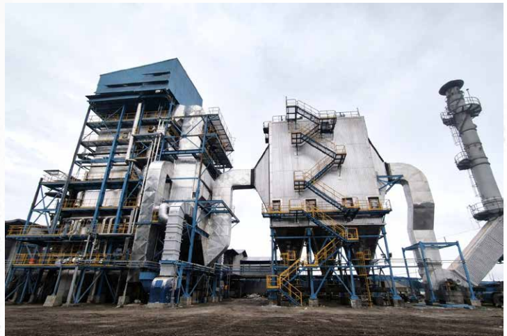
The 1 X 39 TPH Flexisource™ boiler installed at the palm oil producer industry
