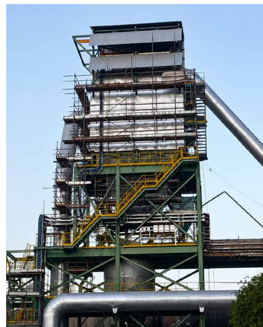
The alkali bypass system installed at the cement manufacturing facility in Thailand
