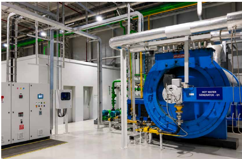
The 30-lakh kcal/hr gas-fired hot water generator installed at the automotive manufacturer in Talegaon, Maharashtra
