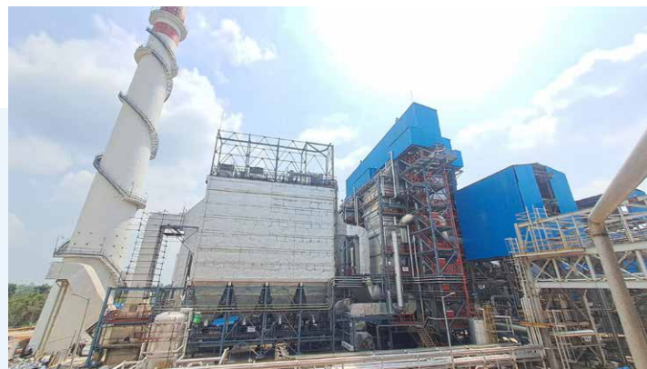
The 2 x 46 TPH reciprocating grate boilers installed at the ethanol biorefinery
