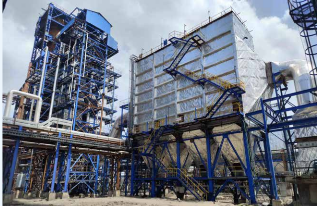
The 2 x 40 TPH waste heat recovery boilers (WHRBs) downstream of 2 x 350 TPD sponge iron kilns installed for the steel manufacturer
