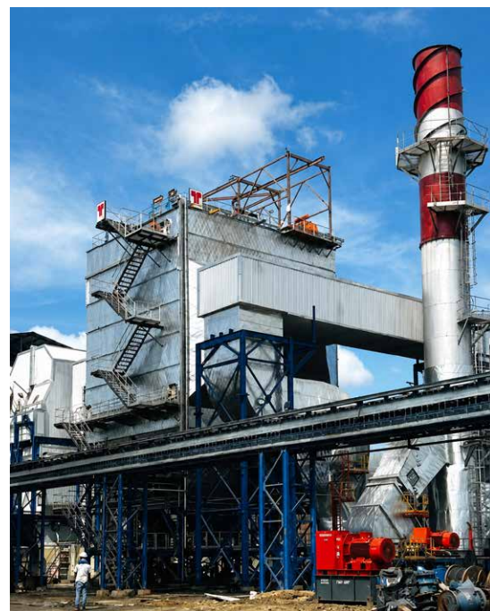
The state-of-the-art electrostatic precipitator installed at the sugar manufacturing plant in Tanzania
