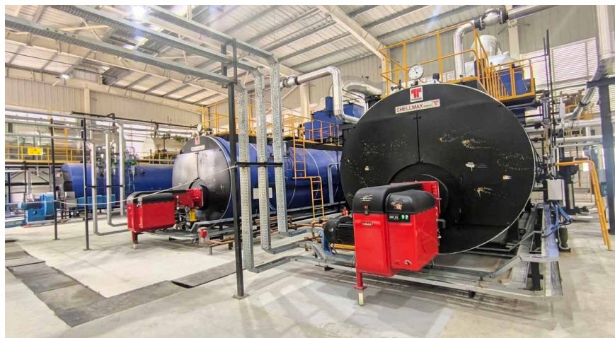
Thermax's boilers installed at the site
