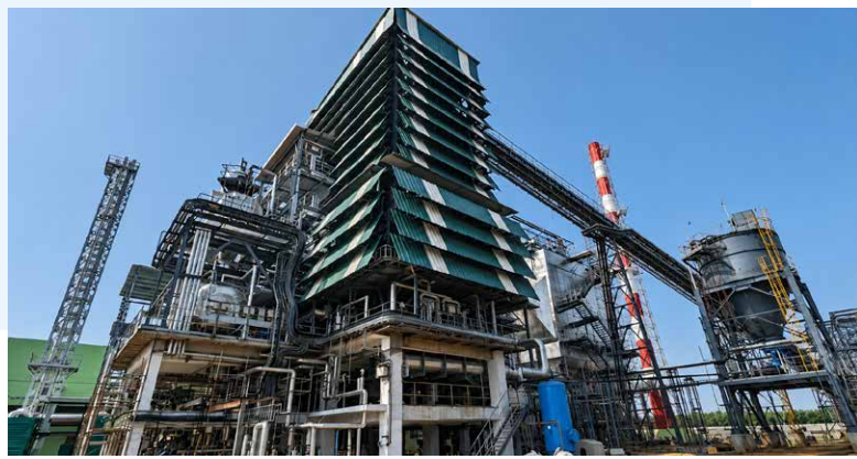
The 1 x 40 TPH AFBC boiler installed at the food-processing site
