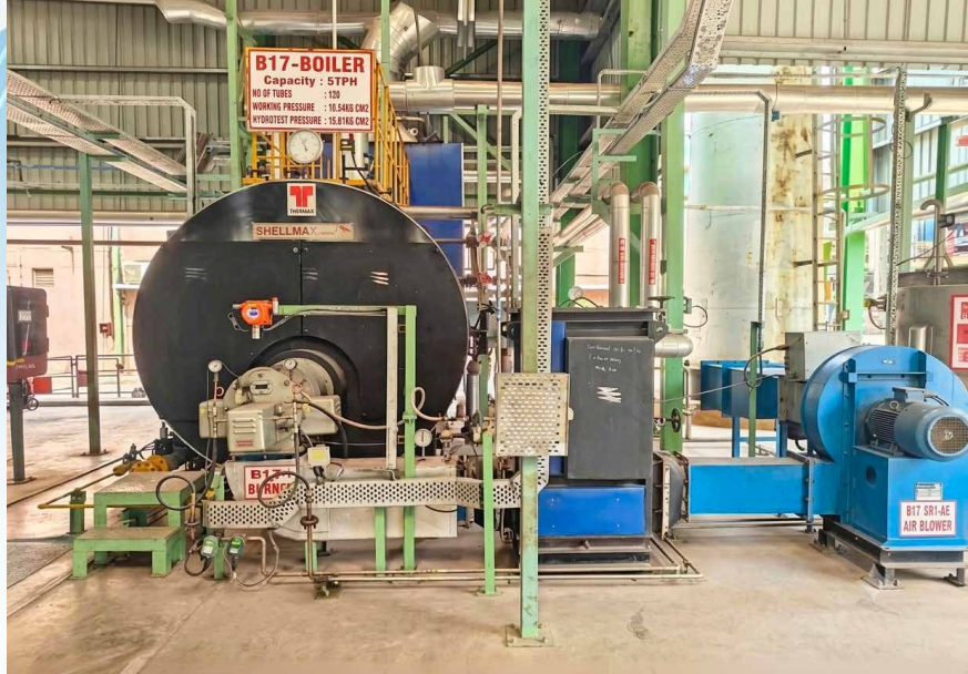
The 5 TPH Shellmax Global Ultra multi-fuel boiler installed at the facility
