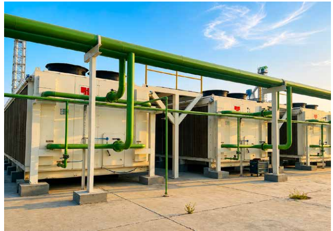
The adiabatic cooling towers installed for a snacks major
