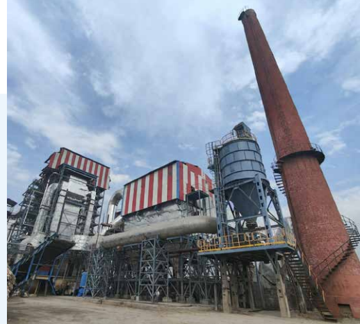
The 1 x 40 TPH waste-to-energy boiler installed at the paper products manufacturing site
