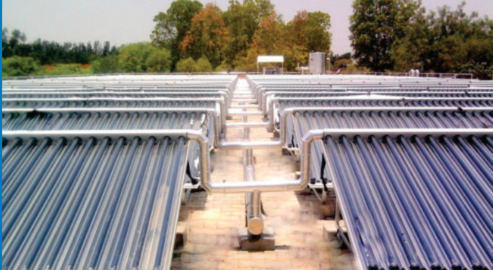
SolPac™ NI30 Collectors for Water Heating Application at reputed FMCG Major, Bangalore
