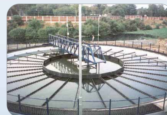
Pimpri Chinchwad Municipal Corporation, Pune 15 MLD
