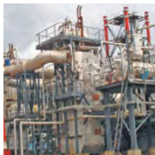
Tank Farm heating
