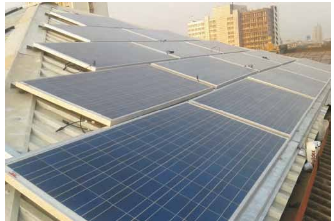
The solar photovoltaic installation for lighting at St. Xavier's college Mumbai, is one of the several aesthetically executed projects from Thermax that are synchronised with the power grid.
