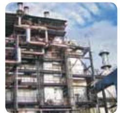
Air pollution control
