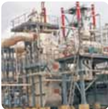
Tank farm heating
