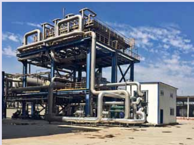
A heat pump installed in China: energy efficiency in industrial applications
