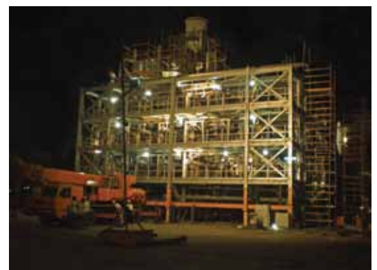
A Thermax waste heat recovery system : meticulous execution
