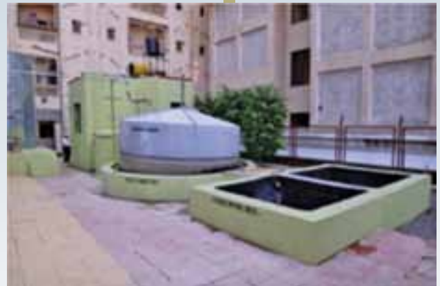
Bioenergen: cooking gas, power and manure.
