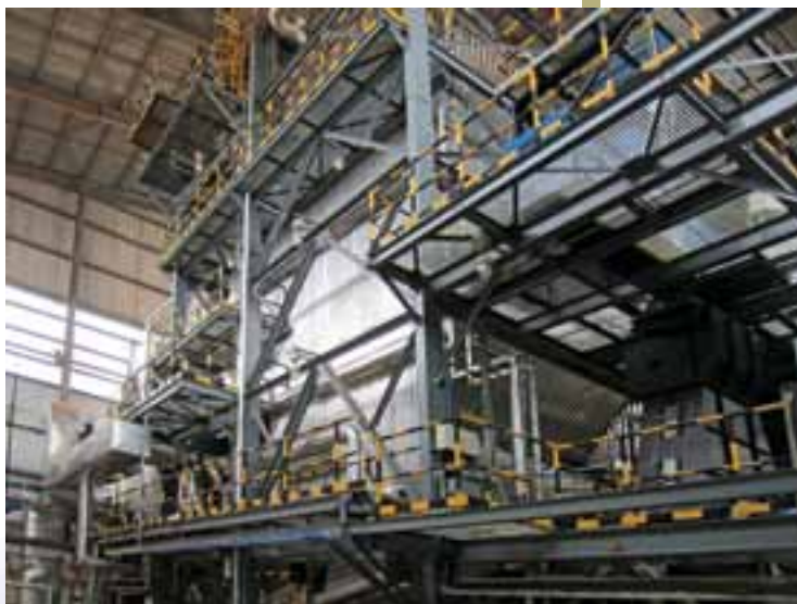
Co-generation boiler at Congo: meticulous project execution
