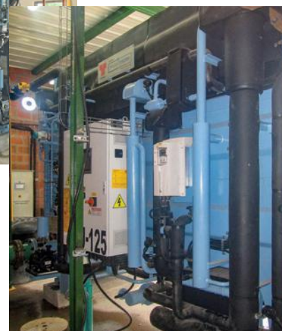
Steam-fired chiller supplied and commissioned for a refinery
