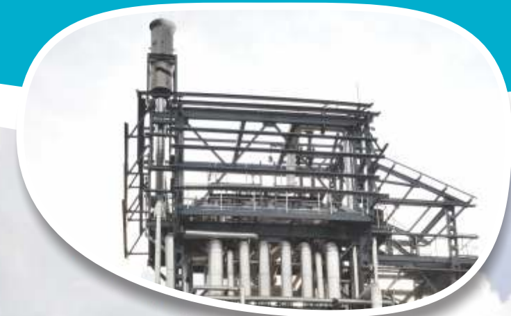
Spentwash fired boiler installed at Bannari Amman Sugars, Karnataka, India
