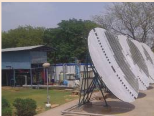
At MNRE's Solar Energy Centre, Gurgaon : integrating solar and biomass
