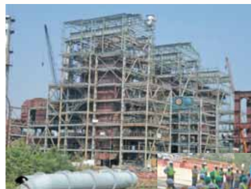
Captive power plant for SAIL Rourkela under construction and (inset) safety pledge at site : presence in PSUs
