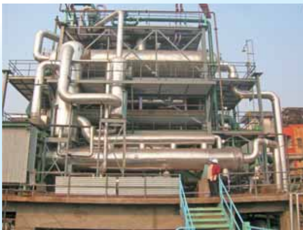
Thermax boiler for sugar industry : Thai installation
