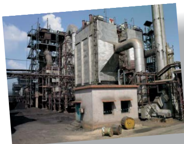
A small power plant : real benefits
