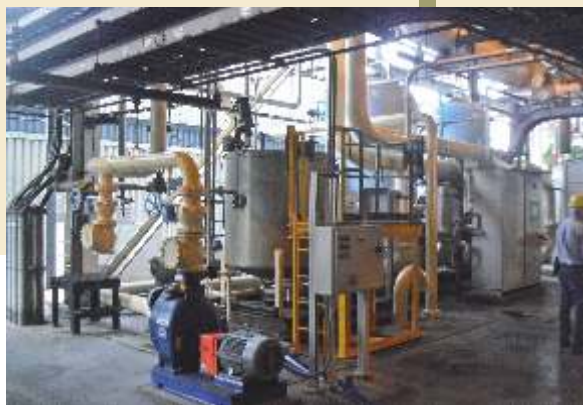
A Graver water installation : water treatment in mega power plants
