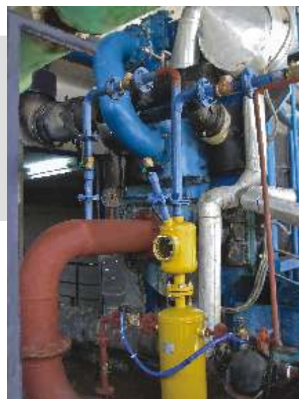
ATCS System : preventing expensive downtime
