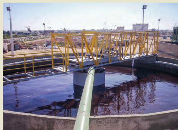
Effluent treatment plant of 1800 m 3 / day at Alexandria Fabrics, Egypt.
