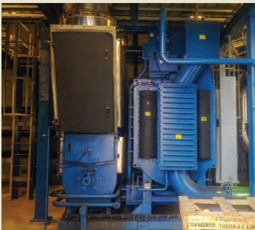
Vapour absorption chiller for process cooling at Guinness Brewery, Nigeria. The 700 TR chiller is driven by exhaust gases.
