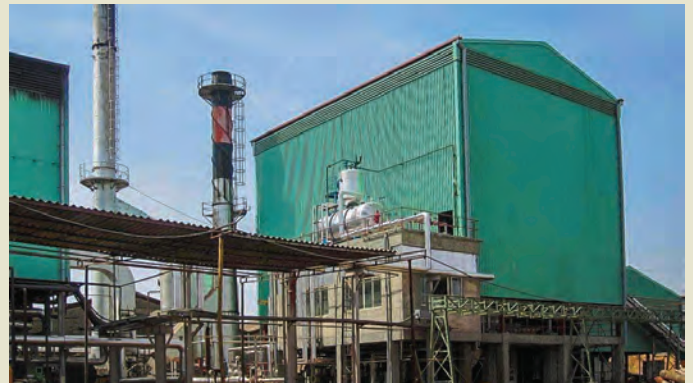
Trigeneration boiler at Bidco, Kenya. The biomass fired boiler provides 20 TPH steam, 2.2 MW power and 400 TR chilling.
