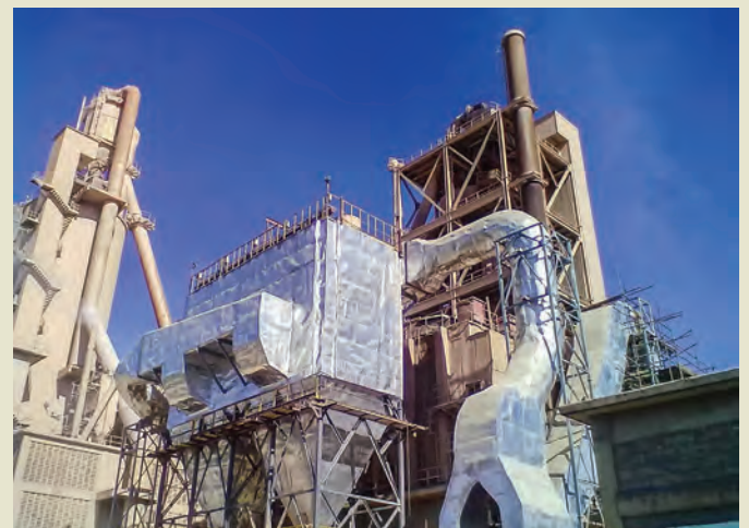
Air pollution control system at Mbeya Cement Company in Tanzania. The 202127 Am 3 /hour pulse jet bag filter cleans the raw mill waste gas.
