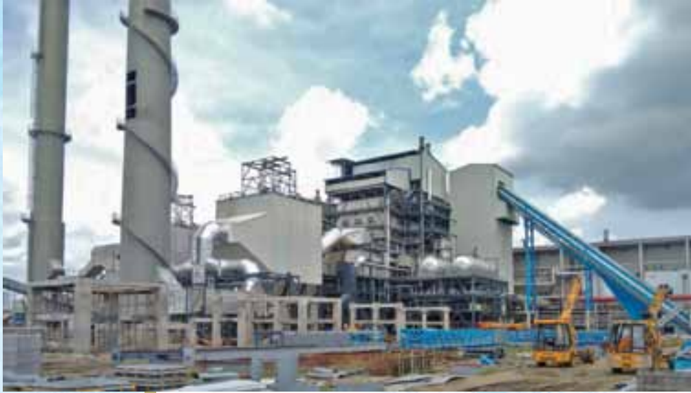
The ICPL plant : sugar and power from a single source
