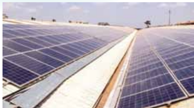
The 1MW rooftop grid: sustainable PV solutions
