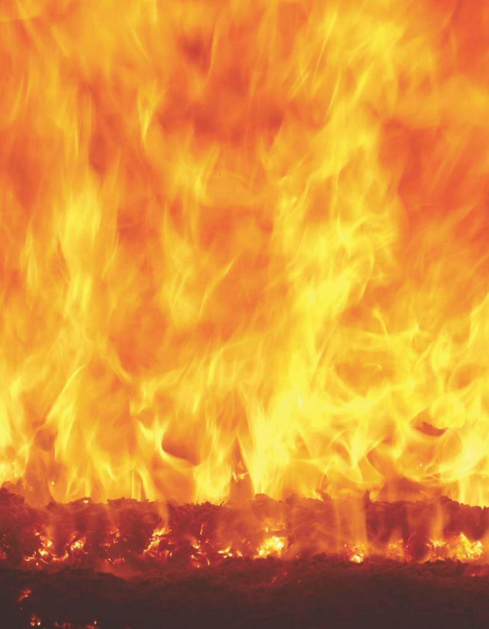
State-of-the-art, reciprocating grate, biomass combustor technology from Lambion, Germany, in operation at a TOESL managed boiler site
