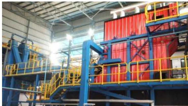
8-ton biomass boiler plant and 6m 3 /hr water treatment plant on Build Own Operate model
