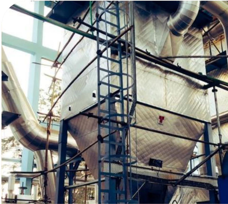
Pulse Jet Bag Filter (PJBF) for a customer in the pharmaceutical industry, installed on a biomass fired boiler
