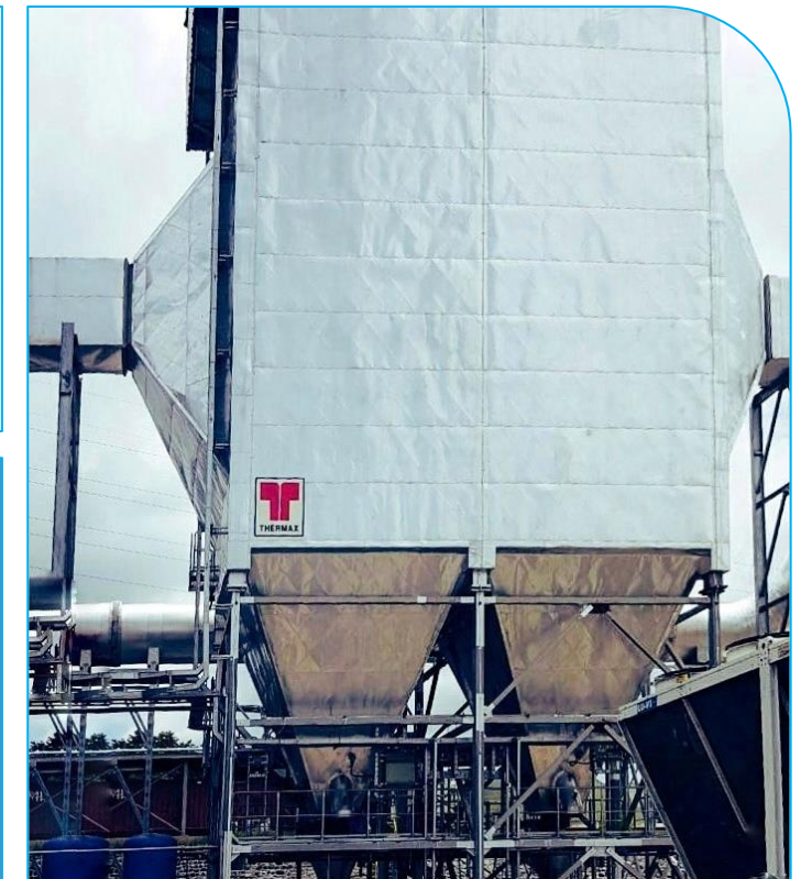
Remote commissioning of an ESP on a husk fired boiler in the Philippines
