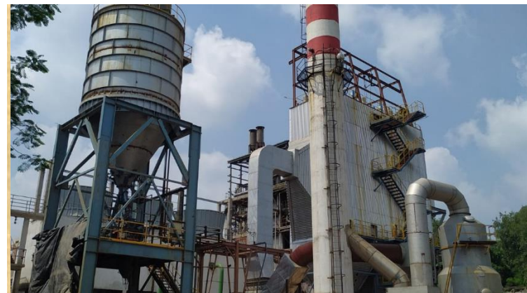
4.9 MW captive cogen plant for a global textile conglomerate
