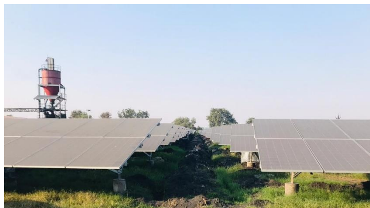
1.25 MW ground mounted solar PV power plant for a leading edible oil manufacturer
