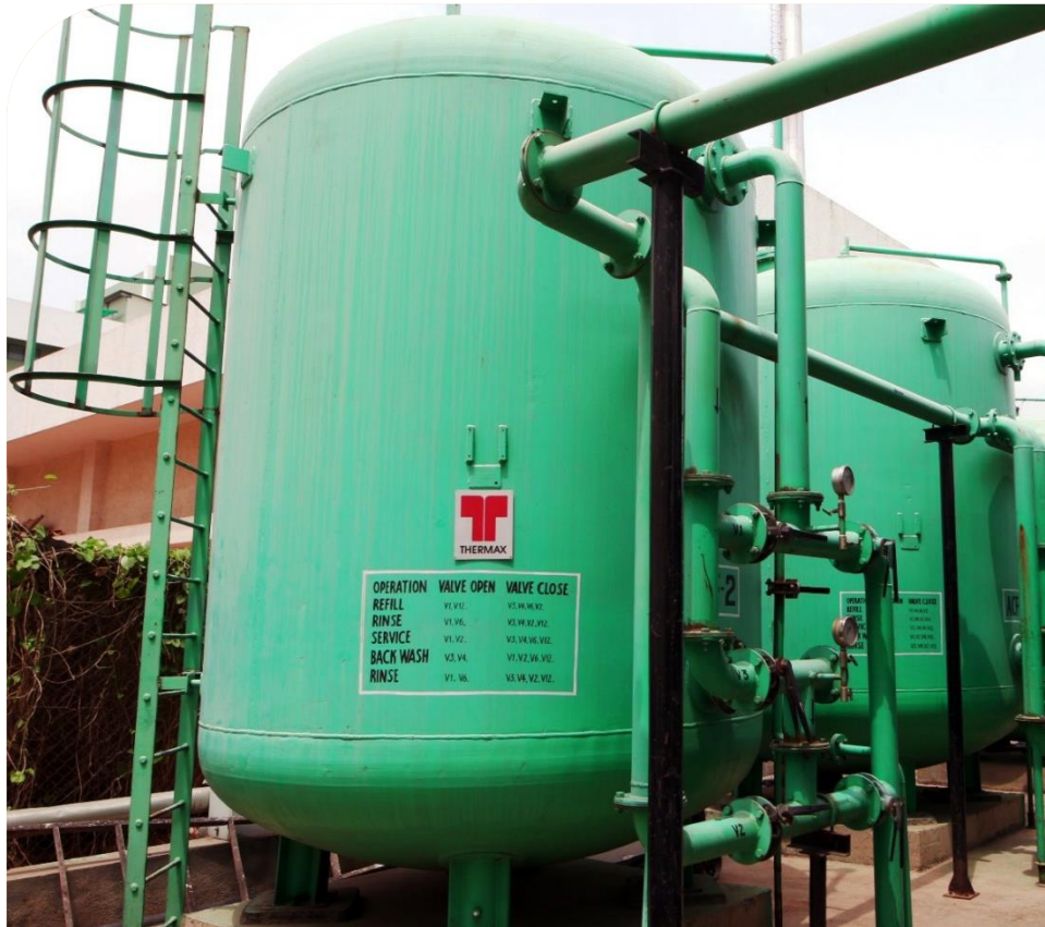
Resins order for Demineralisation plant
