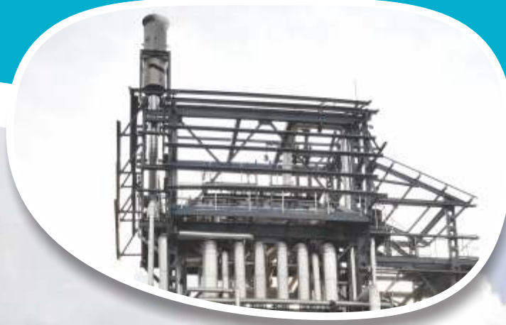
Spentwash fired boiler installed at Bannari Amman Sugars, Karnataka, India
