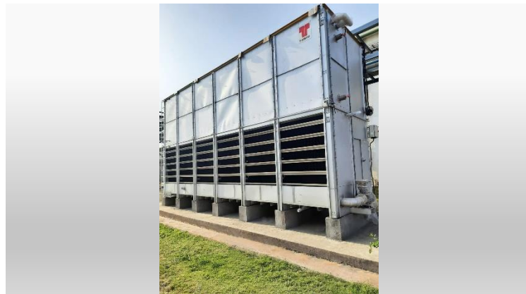
Two Closed Loop Cooling Towers (CLCT) for a global major in specialty films manufacturing
