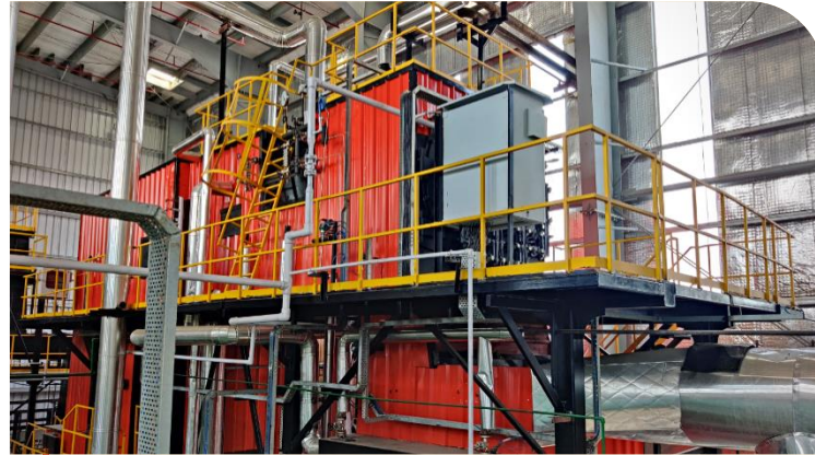
Green steam supply to a tyre major under the Build-Own-Operate model using 18 TPH boiler
