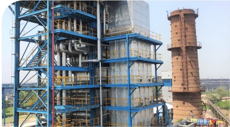
15 MW waste heat recovery power plant for a steel major in eastern India
