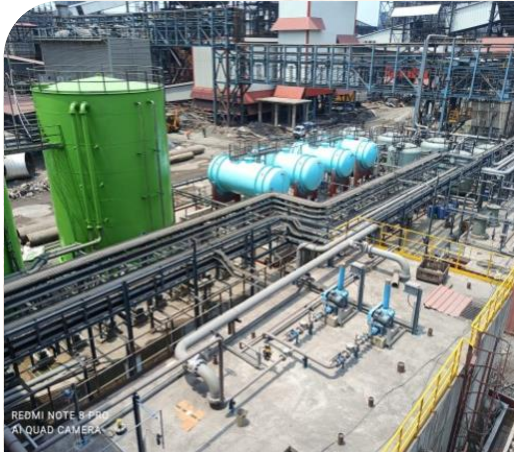
Pre-treatment Demineralisation plant for a steel major
