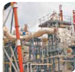
Tank Farm Heating
